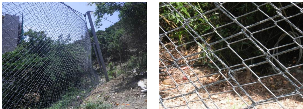
Figure 1: A flexible barrier setup at the Hong Kong University of Science and Technology
