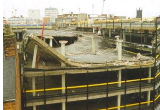
(b) Progressive collapse of Pipers Row Car Park [2]
