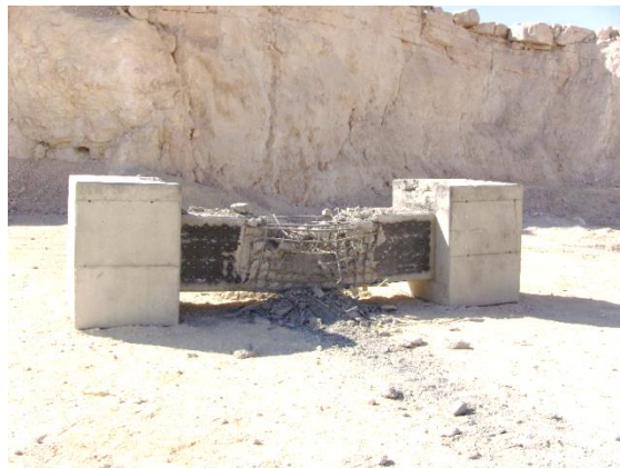
Fig. 1: Severely damaged column due to contact charge
